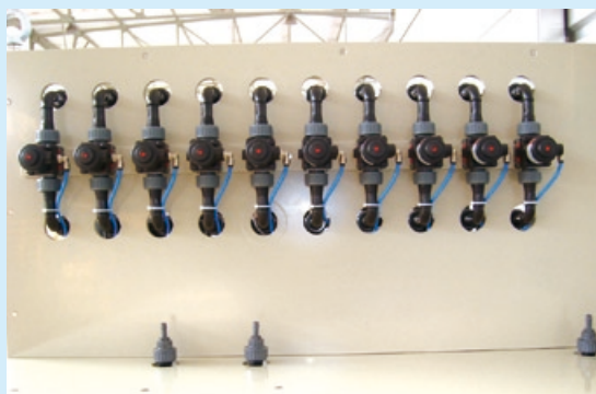
Work space including module-connectors and valve access.
